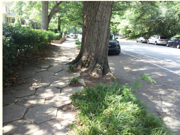
Uneven sidewalk surfaces due to tree encroachment
